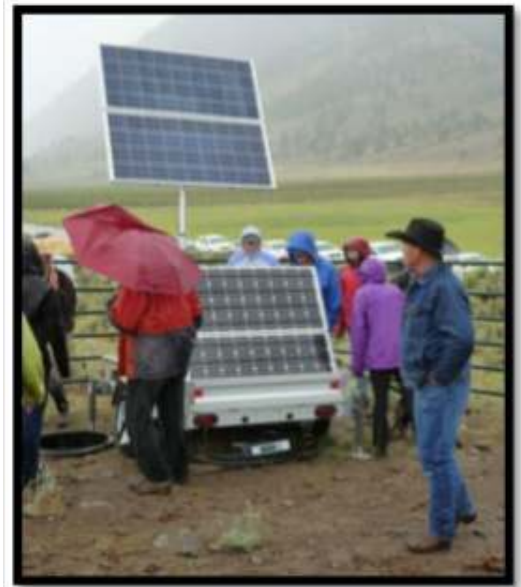
Checking out the mobile solar pump system
